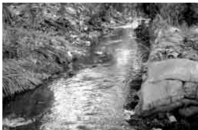
Drainage channels in developing-world coastal cities—like this one in Dar es Salaam—are frequently blocked, leading to flooding
